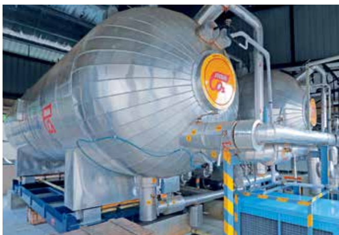
Environmentally friendly carbon dioxide plant at Ceylon Cold Stores, Ranala
