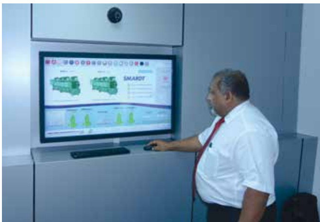
Newly commissioned Building Management System at Cinnamon Grand Colombo
